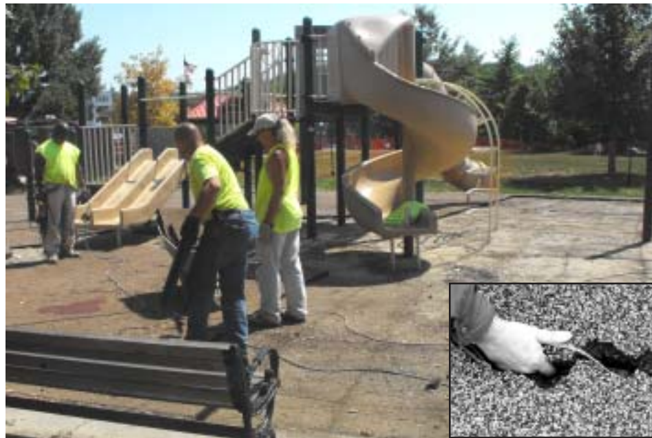
Recreation Department workers remove rubber matting at Hoffner Park. The rubber mat, under the play area was about 10 years . The photo, lower right, shows a tear in the mat and was taken by METRO in the spring.
